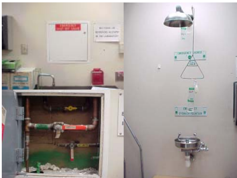
Water and Gas shut off valve and emergency shower and eyewash.
